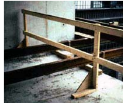
This guardrail appears to be properly constructed except for the missing toeboard that is required to prevent object from falling to the floor below and possibly striking another worker.
