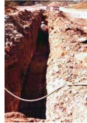
This worker is in a trench with no protective system, that is not sloped or benched and has no means of egress.
